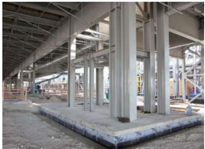
Inside the Cargo Warehouse - Steel Columns on a pile cap with pile foundation
